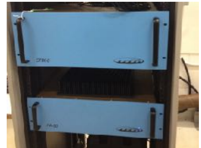
HFR Power Amplifier and Rx
